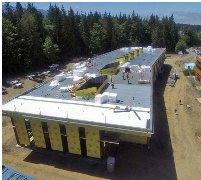
Aerial View of Allied Health and Early Childhood Development Center under construction
